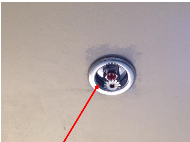
Semi-recessed head with less than 1/2" clearance below the ceiling surface
